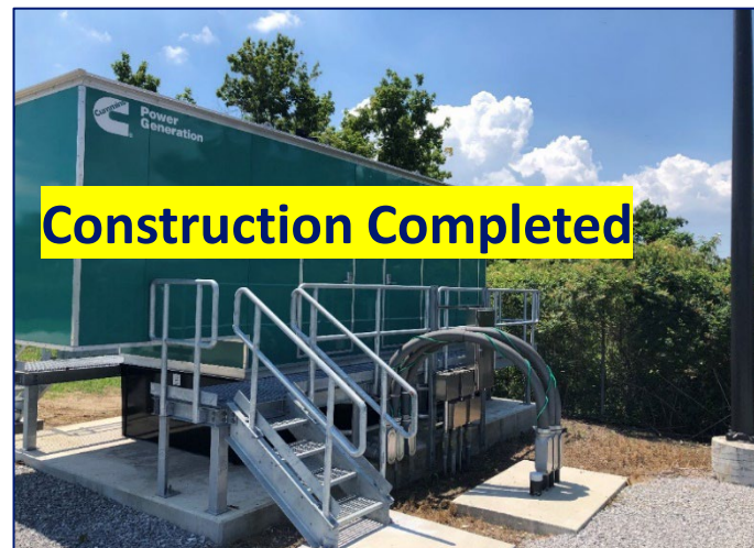
Lake Timberlane New Lift Station & Generator ($2.6 Million)
