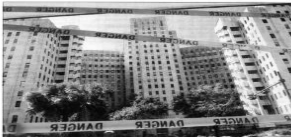
CAUTION Caution tape warns people away from Charity Hospital. Damage from Hurricane Katrina has left the hospital unusable, teeming with not only mold but also potentially lethal bacteria. STAFF PHOTO BY NAIT POPE
